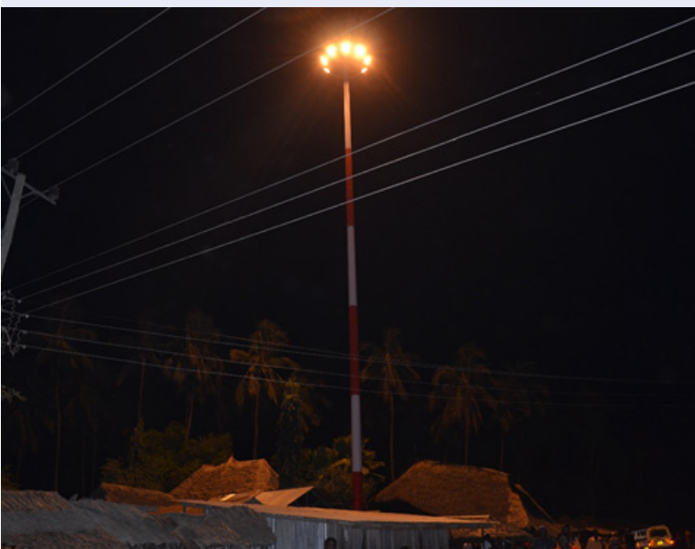
Tezo Township Highmast Lighting
